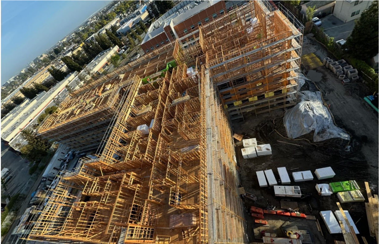
Figure 1 – Framing progress at the northern building, April 2024. This building is framed up to the fifth story and window installation is in progress.
