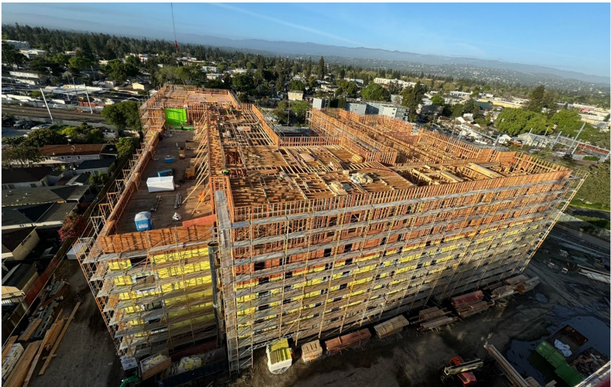
Figure 2 – Framing progress at southern building as of early April 2024. This building is completely framed up to the fifth story. Windows are installed up to the third story. Level six framing and roofing are in progress.
