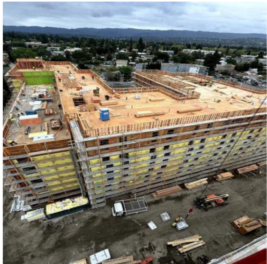
Figure 2 – Wood framing progress at the southern building, May 2024. This building is framed through the roof. Windows are installed through the 4th story.
