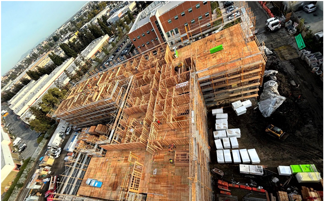
Figure 1 – Framing progress at northern building as of early March 2024. Certain sections of this building have walls completely framed up to the sixth story.
