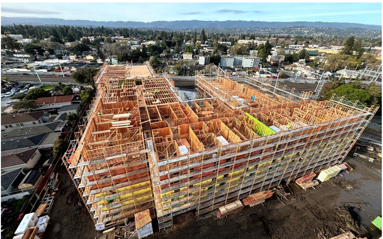
Figure 2 – Framing progress at southern building as of early March 2024. Certain sections of this building have walls completely framed up to the fourth story.
